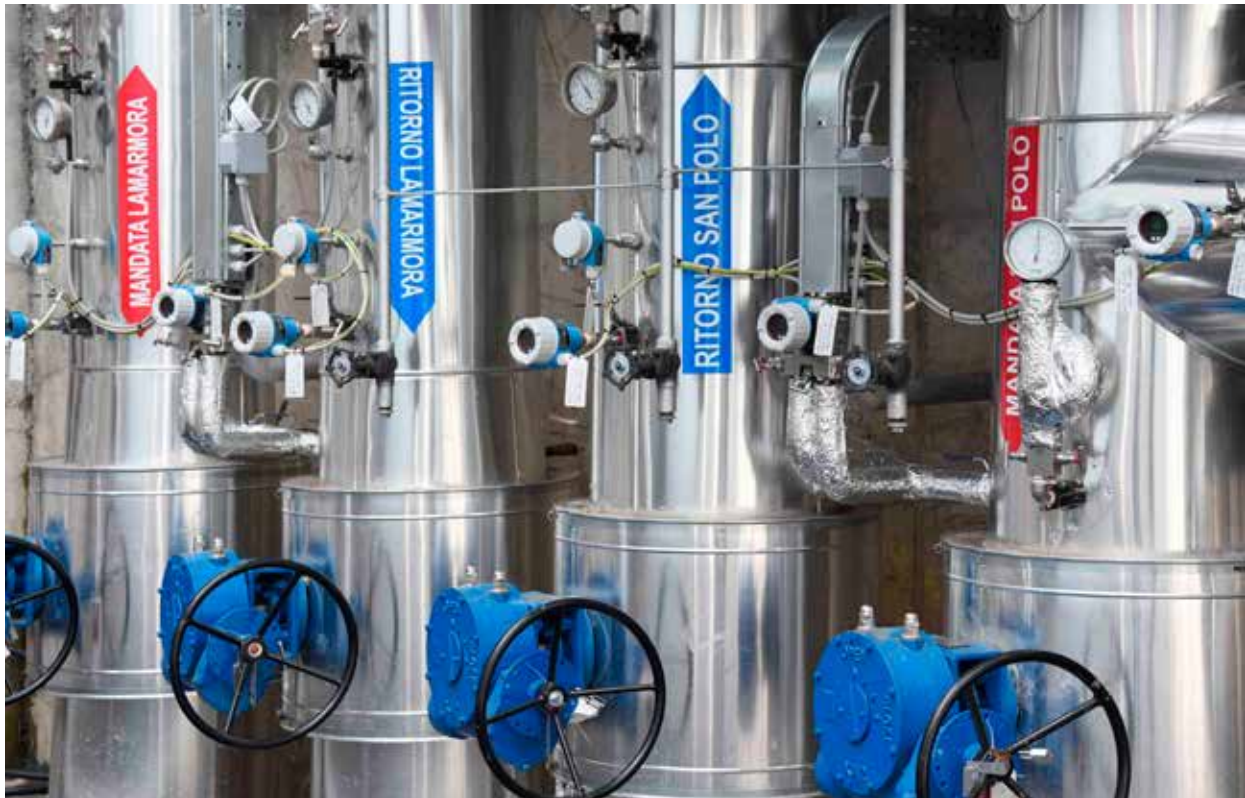
Close-up of the interconnection hub with the district heating network
