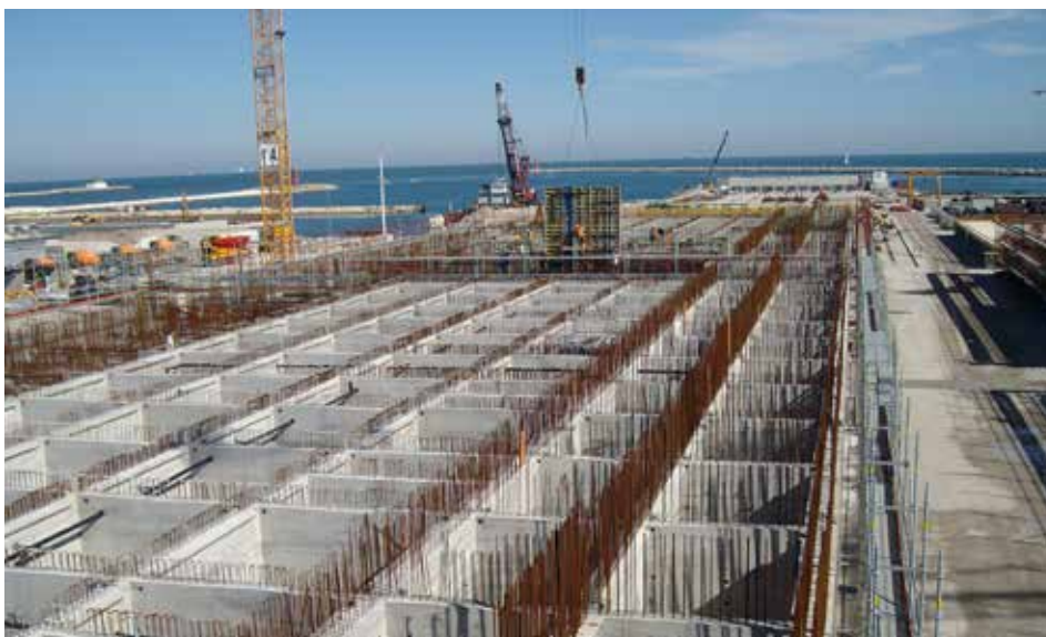
Venice Malamocco harbour pass. Construction of the structures forming the foundations of the MO.S.E. system that was conceived to protect Venice from sea-level rise. The four barriers are now completed.
