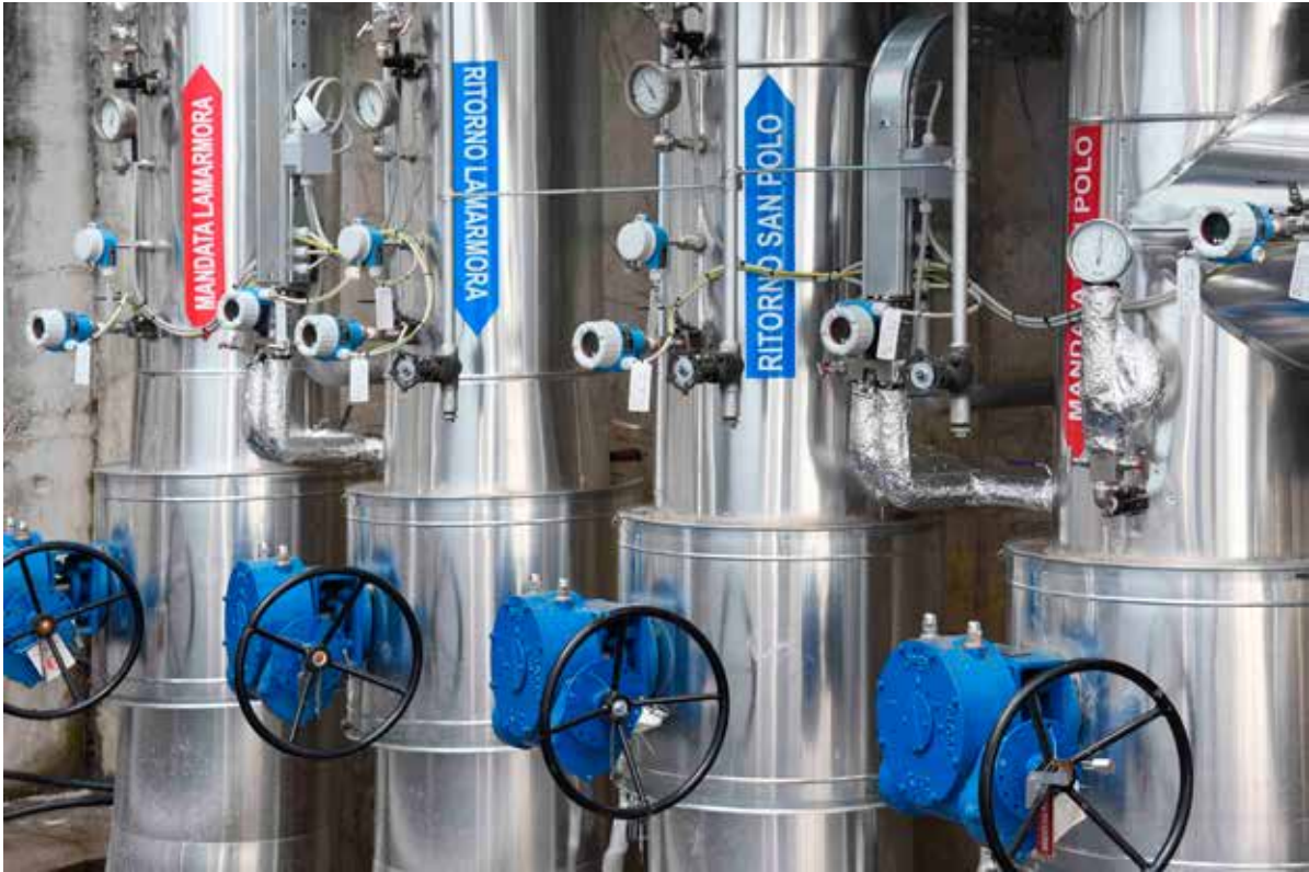
Close-up of the hub interconnecting with the district heating network.
