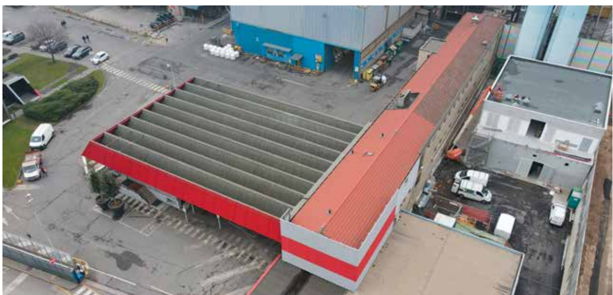
Works in progress for the construction of the heat recovery plant in 2020
