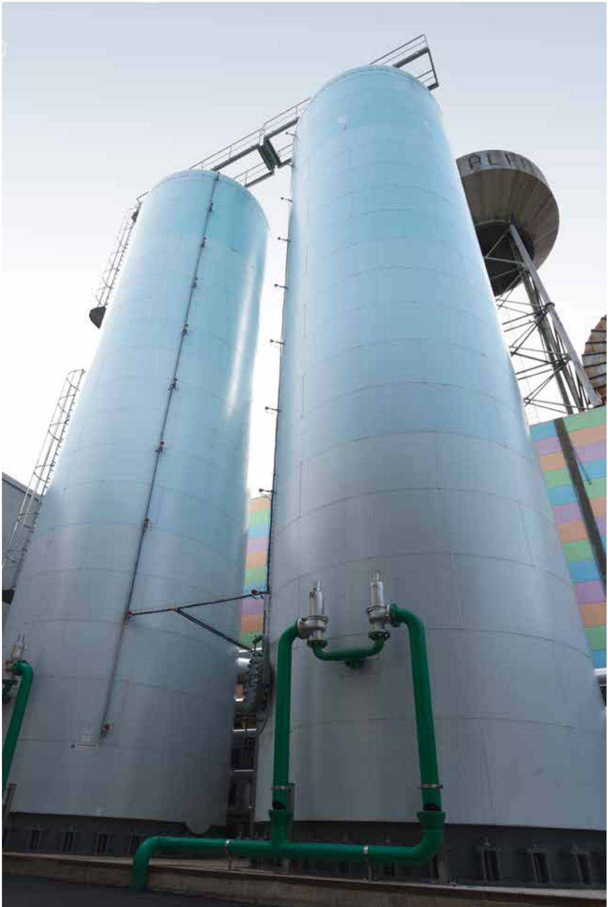
Hot water storage tanks serving the heat recovery plant
